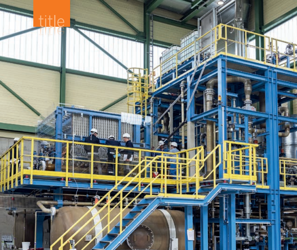
Looks complicated, but benefits the energy transition: hydrogen is produced in an electrolyser.
